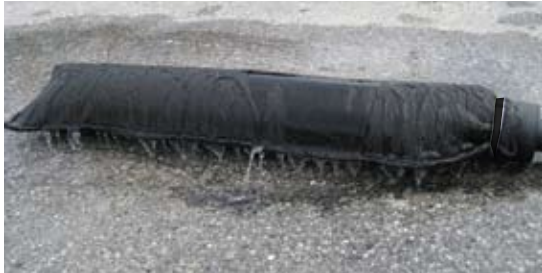
EVAC Filtration System filtering water.
